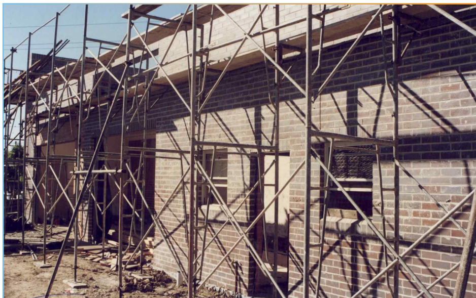
Below: SDN Hurstville during construction, 1996. The front section was kept but the rest was rebuilt. Source: SDN Archive
